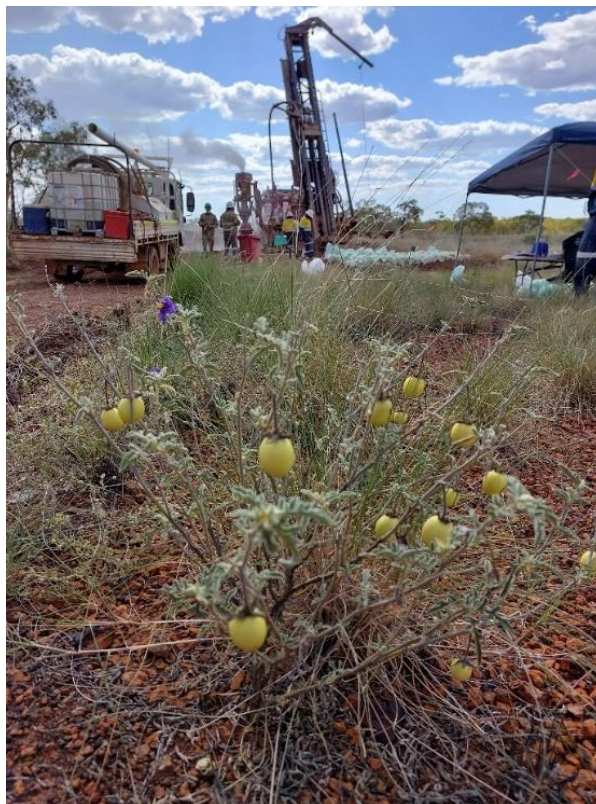
Figure 7. Tulla RC rig TD04 drilling BURC00686 to south of Anthill open pit.
