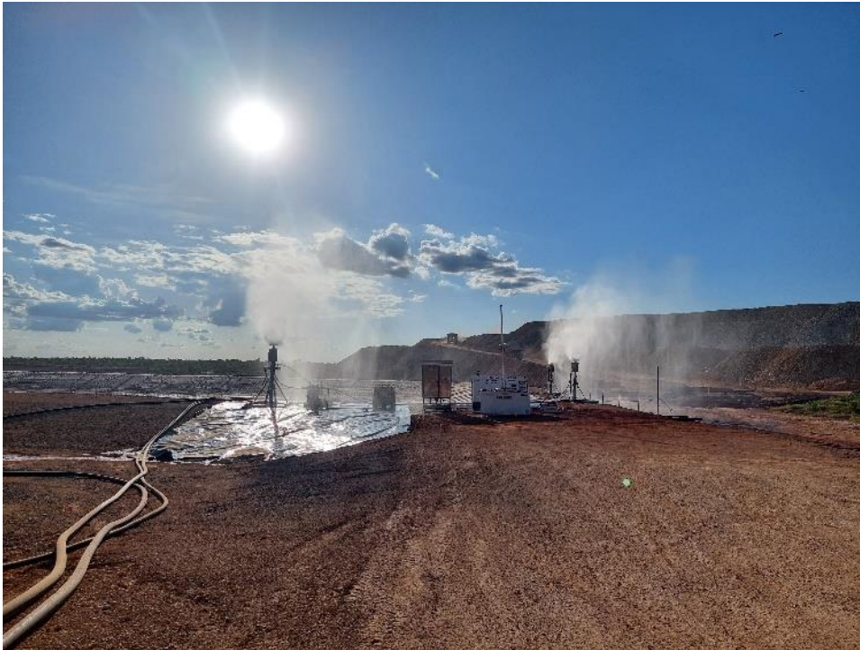
Figure 1. Evaporators form part of Austral's water management.
